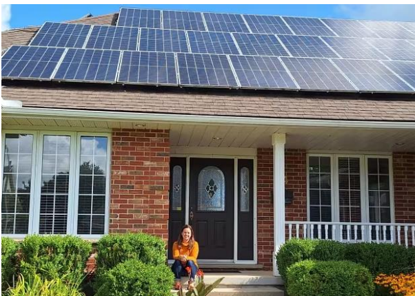
Figure 5 Example of a roof-mounted solar photovoltaic installation
