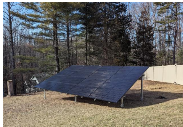
Figure 6 Example of a ground mounted solar photovoltaic installation
